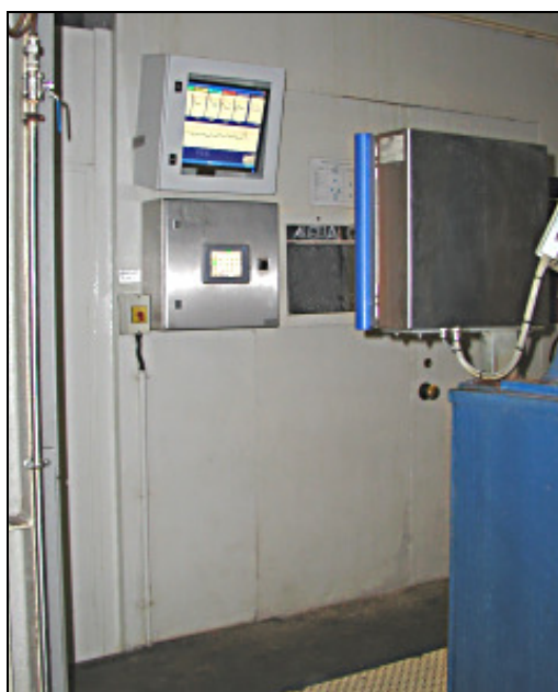
Figure 2. Display monitor and automatic water spraying control unit.
