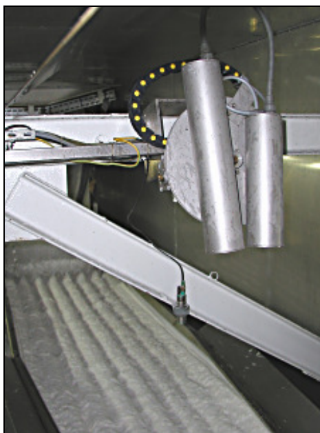
Figure 1. Measuring unit installed over the wet sugar 'grasshopper' conveyor.
