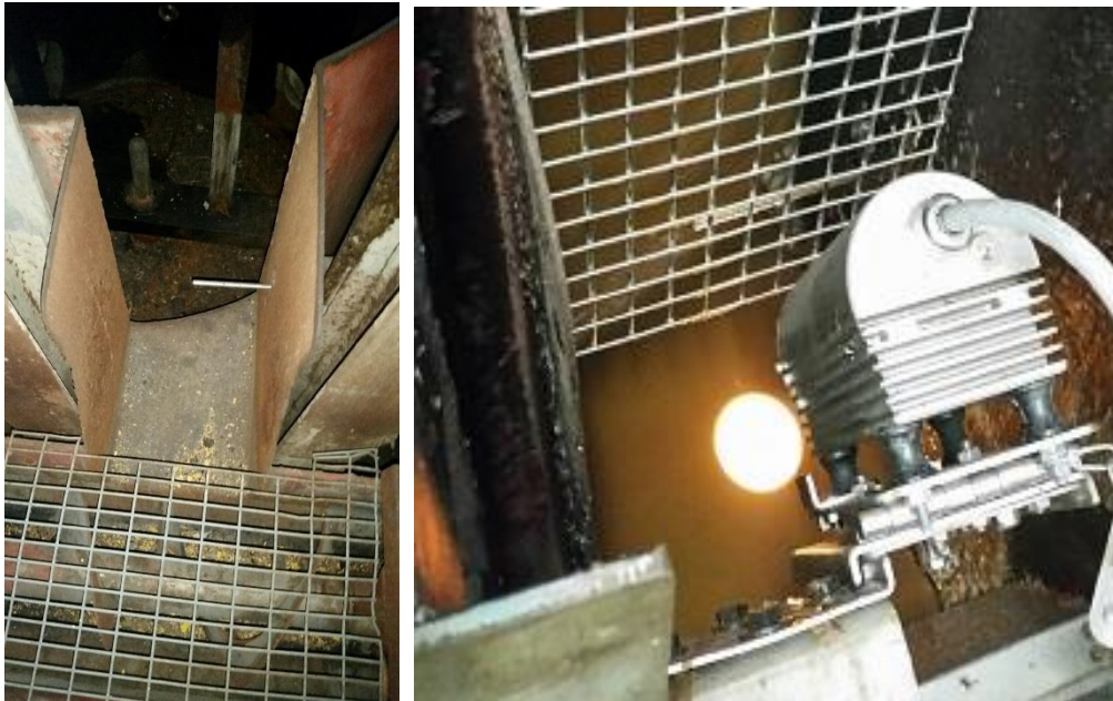
Figure 2. Transition from Magma Screw to Tank and Neltec unit in position.
