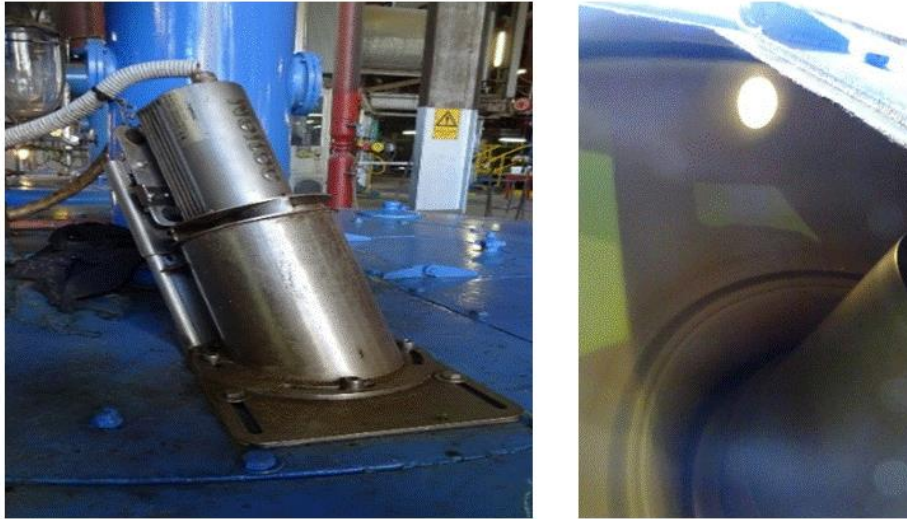
Figure 7 The Neltec transducer on No 4 fugal and the light beam on the basket.
